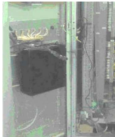
Fig. 7: Signal conditioning box in Abadan utility plant 1 substation
