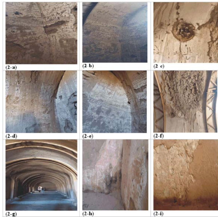
Fig. 2: (from a to I): The status of Pilgrims' Room in the Monastery. a: Murals and paintings in arched rooms along the northeastern corner layers of dirt and dust. Photograph taken in 2019. b: shows a large fragmentation and collapse in the plaster and the writings that are important for the dating of historical events. c: The hives of wild bees are dotted abundantly on the walls. Photograph taken in 2020. d: shows significant fragmentation and collapse in the plaster layers. Photograph taken in 2020. e: shows the inscriptions and writings that will be placed on the entrance walls. Photograph taken in 2019. f: shows the metal supports installed on the walls. With these existing supports, we need to treat the rusty iron left on the walls. g: The corridor goes north-south and contains the monks' rooms. Photograph taken in 2020. h: shows soot spots on the surface and a blood spot from bats. Photograph taken in 2020. i: shows the salts on the surface of the preparation layer, fungal growth in many areas and biological residues.
