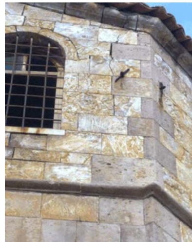
Fig. 5: Cracks on masonry wall
