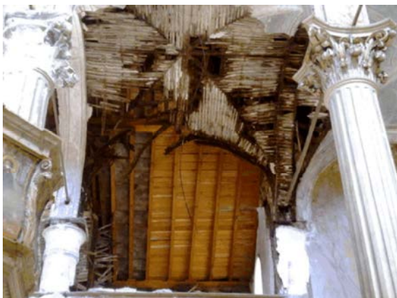
Fig. 10: Roof repair by ignoring restoration principles
