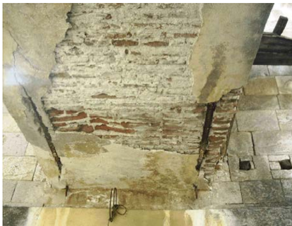
Fig. 9: Iron Reinforcement Heavy Corroded
