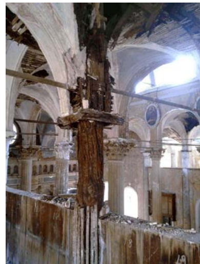
Fig. 6: Damaged Wood Columns
