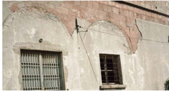
Fig. 4: Gaps made filling with masonry walls between Vertical Columns and Arches
