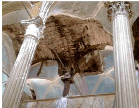
Fig. 11: Status of the damaged roof
