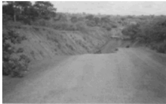
Fig. 5: Eroded sites in Amaokwe Community, Abia State
