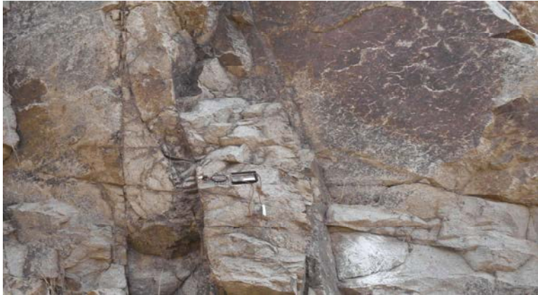
Fig. 4: Fracture as seen on the Basement Complex
