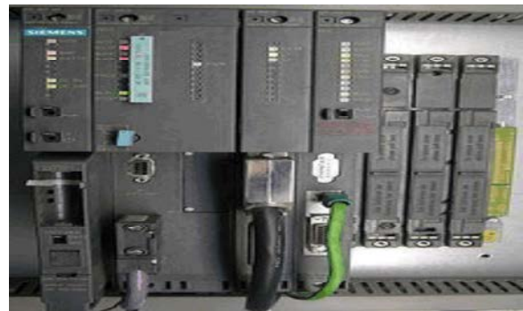
Fig. 2.2: Siemens Simatic S7-400 at Rack 7
