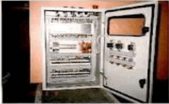
Fig. 2.5: PLC with Control Panel
