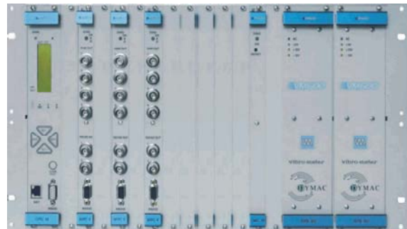
Fig. 1: Non contact probe connection main board in sub station.
