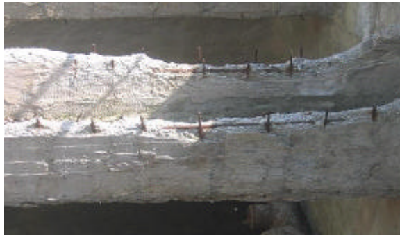
Fig. 1: Damages of reinforced concrete constructions after 35 ± 5 years of exploitation in the condition of environmental activity
