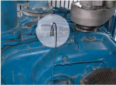
Fig. 9: Typical on line monitoring system of screw compressors [13]
